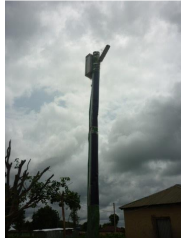
Newly installed solar street light
